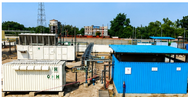
View of Hydrogen Facility
